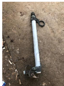
Gambar 4. Fuse Cut Out (FCO) Rusak
