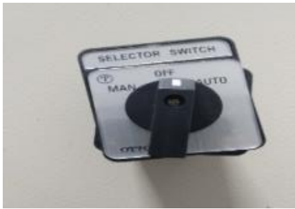
Gambar 6. Main Auto Selector Switch
